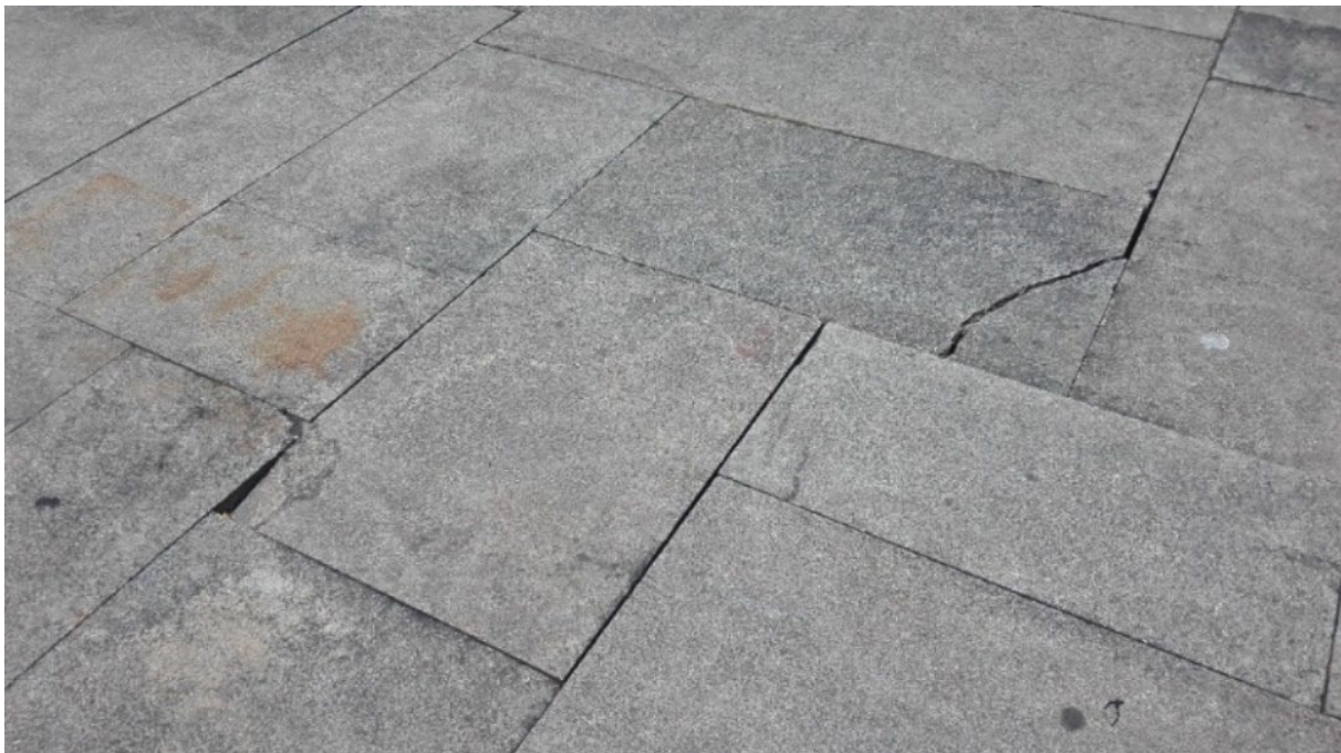
Figure 7: Cracks in the stone floor slabs
