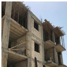
Figure 5. Poor edge protection
