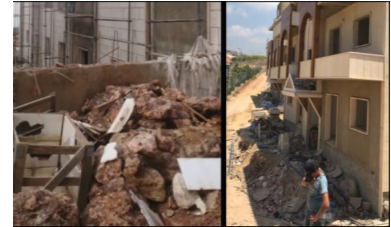
Figure 4. Messy surroundings and improper waste disposal
