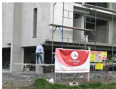
Figure 10. A worker performing plastering without any PPE in a small construction company
